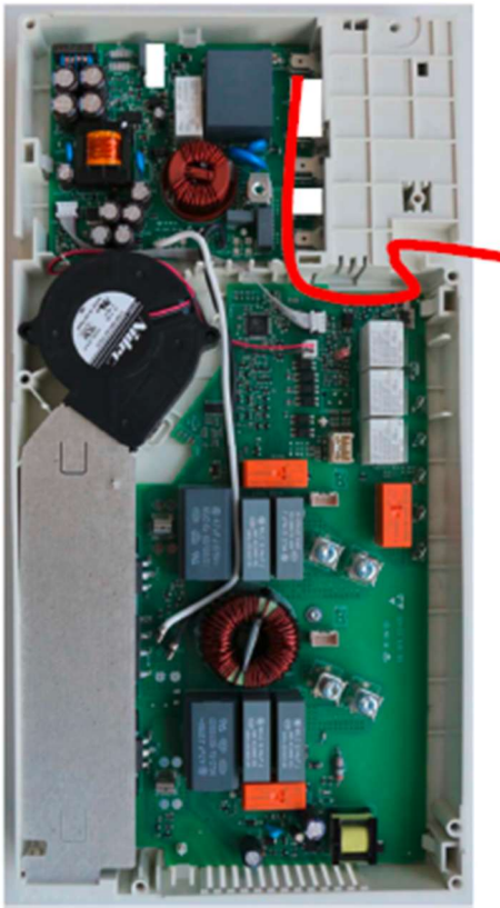
2-burner slave generator (left)
